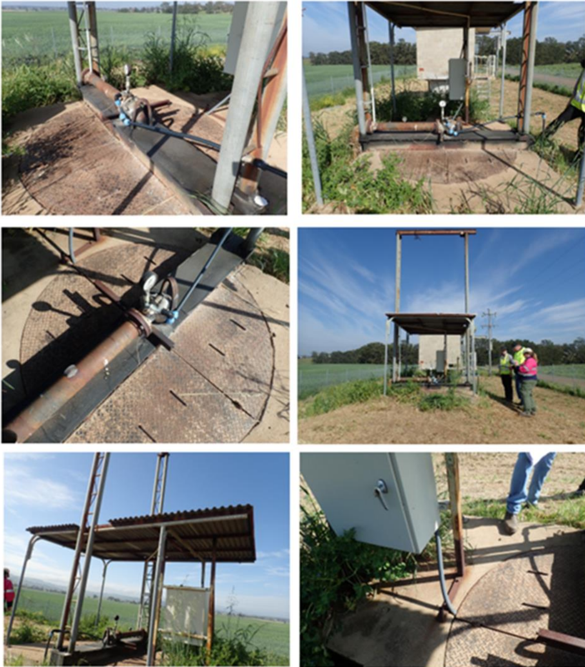
Figure 7 - Coolah Back -up Well
