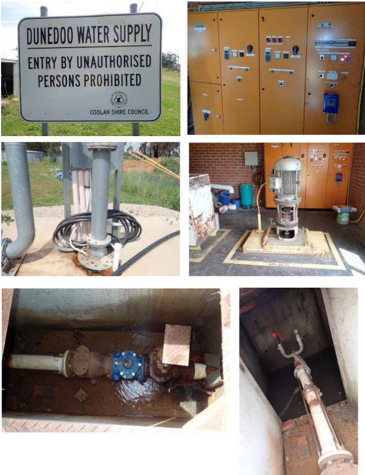
Figure 9 - Dunedoo Town Water Bore
